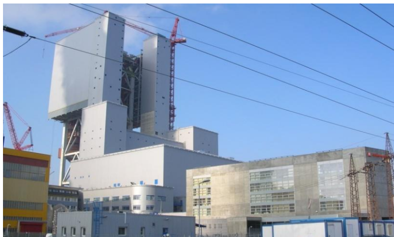
New power resource 660Mw in Ledvice power plant, Czech Republic
